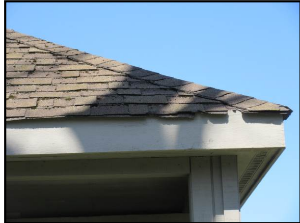
Shed roof with moss & brittle shingles
