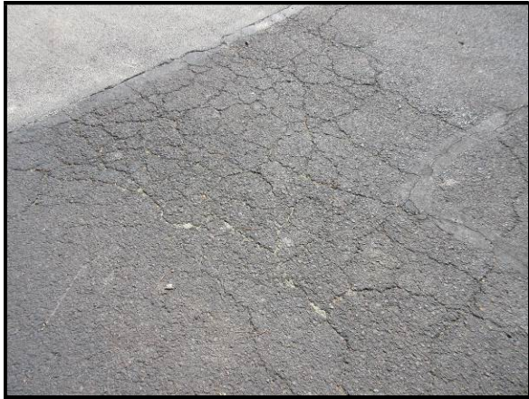
Alligator cracking at tennis court parking area
